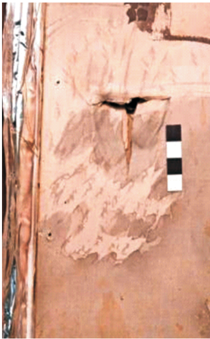
Figure 3. Detached silk exposing the underlying layer and tears in the surface of the silk, evident in different areas.
