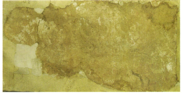
图7 地仗酥碱、颜料层脱落 Fig. 7 The disruption of plaster and the falling pigments
